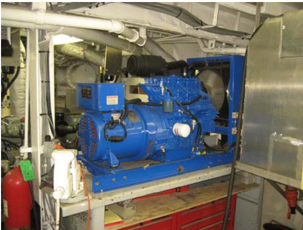
25 kW Backup Genset
