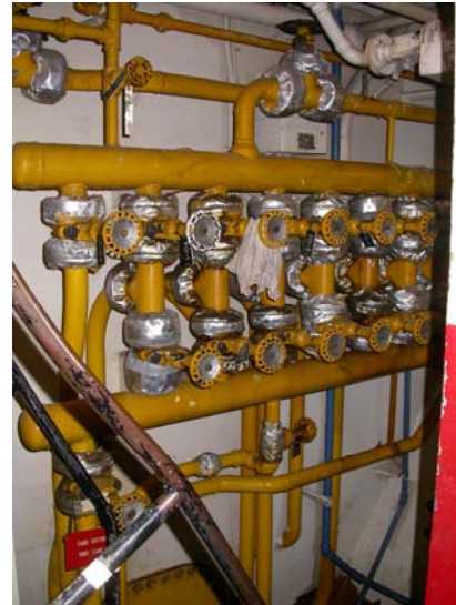
Fuel oil transfer manifold
