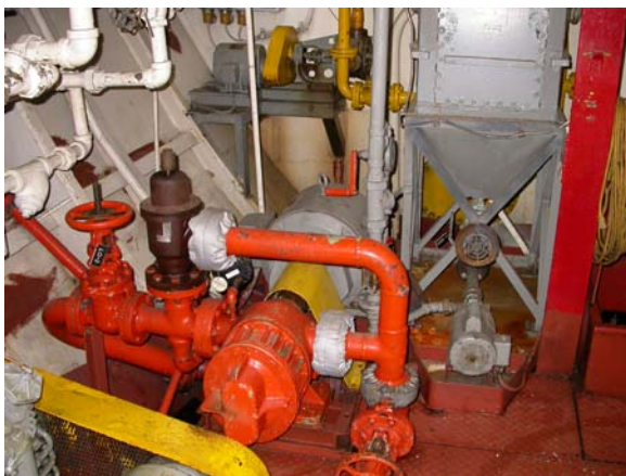
Main engine pre-lube pump
