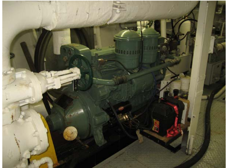
Fire pump auxiliary
